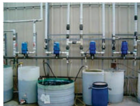
Tanks of fertigation system containing nutrient solutions
